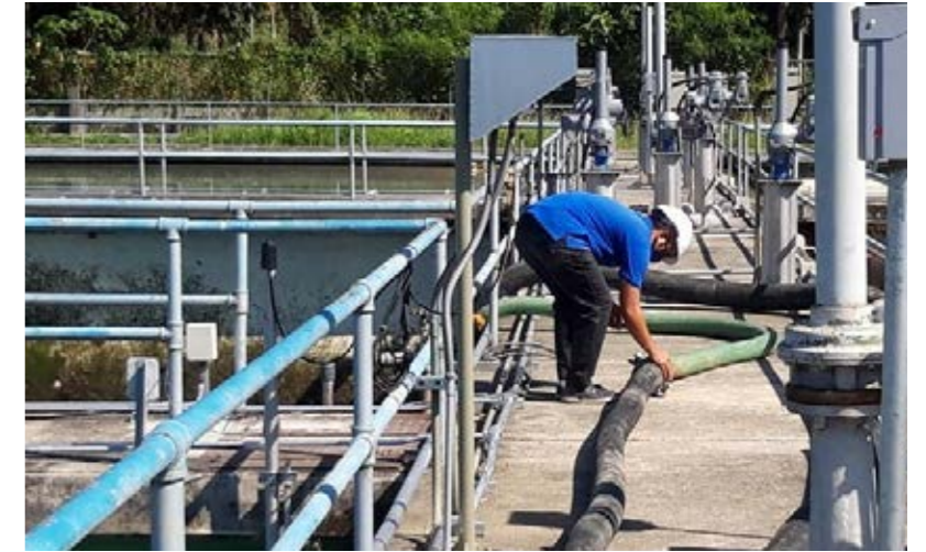
Manila Water continued to improve its facilities despite the pandemic, investing ₱12.1 billion in capital expenditures in the year.
