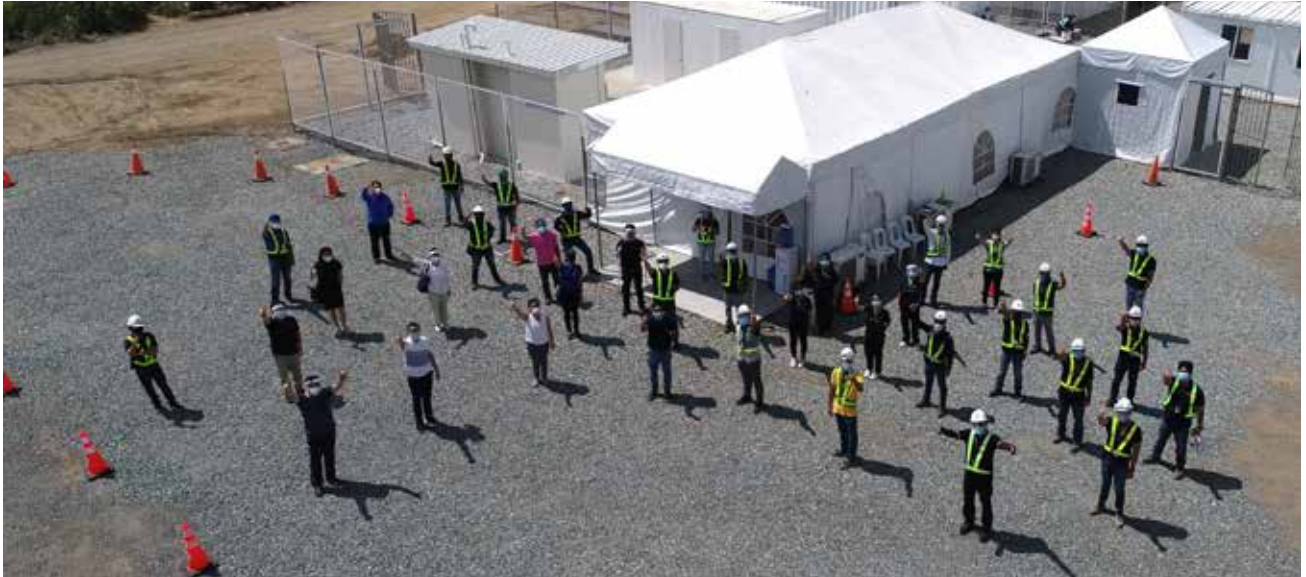
A triage holding area was built adjacent to QualiMed-Sta. Rosa expanding the hospital's capabilities as a full-scale COVID-19 referral hospital.
